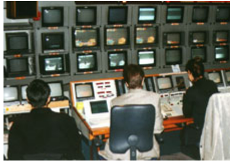
In the control room
